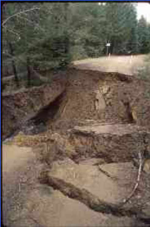
Kelly Rd. bridge collapse
